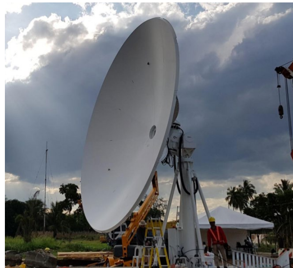
The Davao Ground Receiving Station 7.3-meter satellite tracking antenna in the CAAP Facility, Davao City
