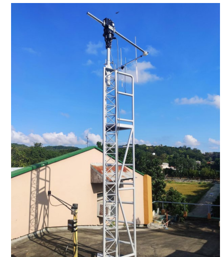
Antenna tower installed in University of San Carlos
